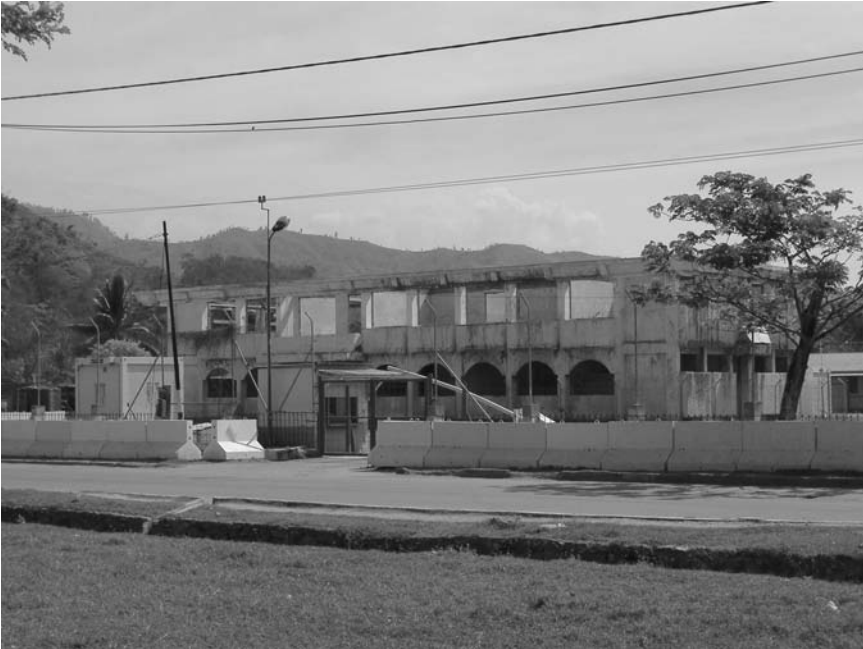
Figure 6.8 Destroyed building in Dili, Timor-Leste.
