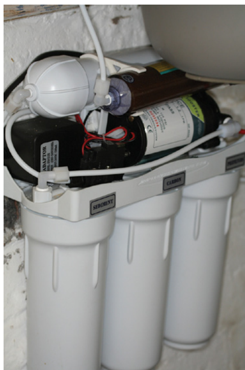
Figure 8.8 Reverse osmosis water unit.
