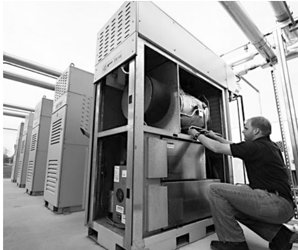
Fig. 8.1 Installation of several 65 kW microturbines
