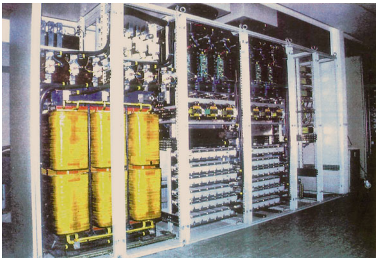
Fig. 10.46 500kVA 12-pulse current source converter
