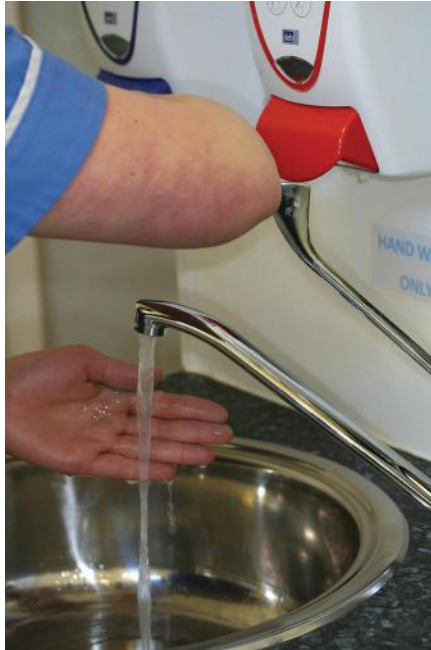
Figure 4.4 Elbow-operated tap in use.
