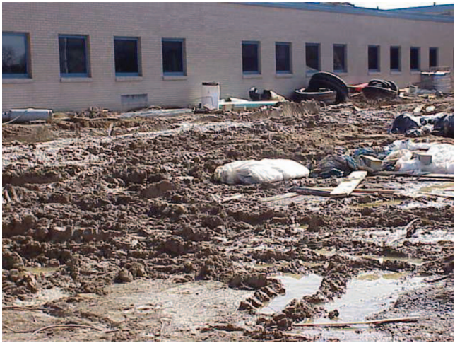
Fig. 5-3. Muddy Site Conditions Caused by Rain and Failure to Seal Exposed Areas
