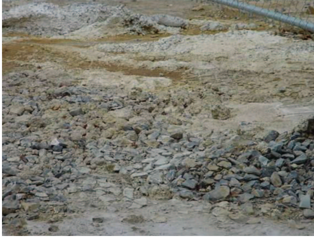
Fig. 5-8. Failed Site Area
