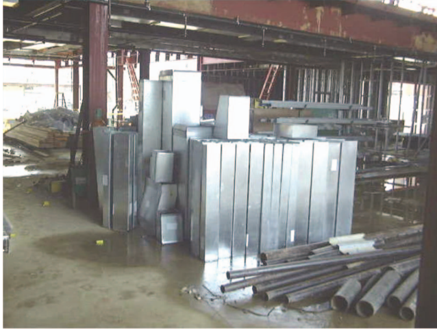
Fig. 11-2. Untidy Work Face Area
