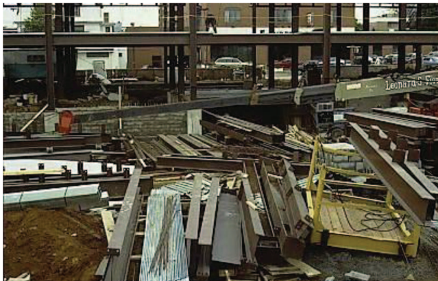
Fig. 6-13. Poor Material Storage Practices, Rider Building, State College, PA
