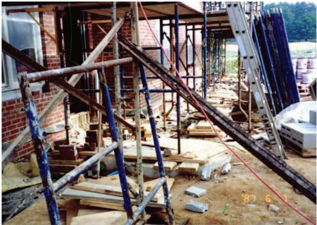
Fig. 6-22. Poor Housekeeping at a Staging Area, Sassafra Project, Selinsgrove, PA
