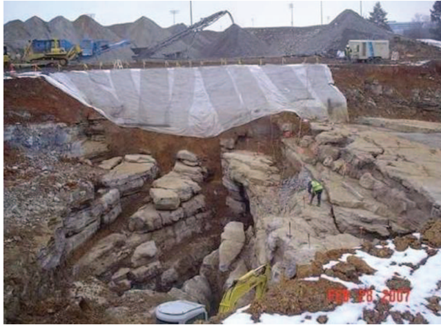
Fig. 11-1. Sinkhole in the Center of the Katz Building
