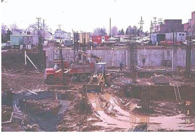
Fig. 6-15. Muddy Site and Storage Conditions, Walker Building
