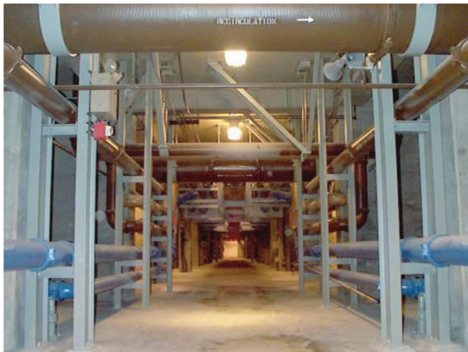
Fig. 12-6. Below-Grade Piping Gallery
