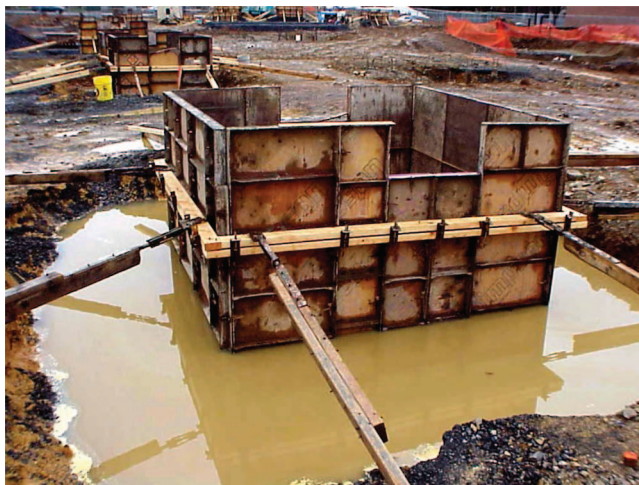
Fig. 5-5. Flooded Footers Caused by Runoff from Off Site
