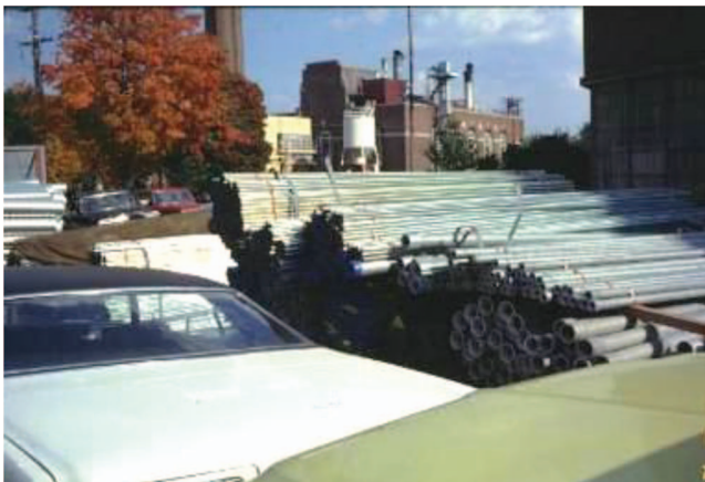
Fig. 6-14. Inaccessibility of Stored Materials, Walker Building
