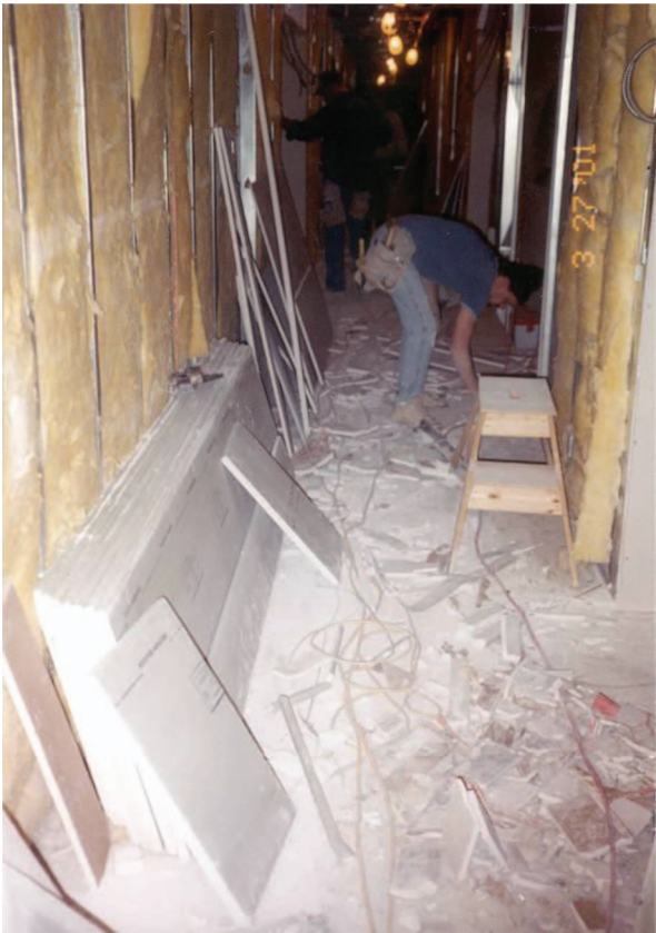
Fig. 6-21. Poor Housekeeping at a Distribution Point, Hampton Inn, State College, PA
