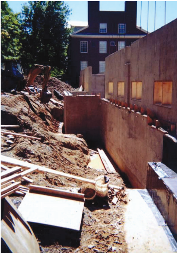
Fig. 8-6. Late Backfilling that Impedes Access to the Building
