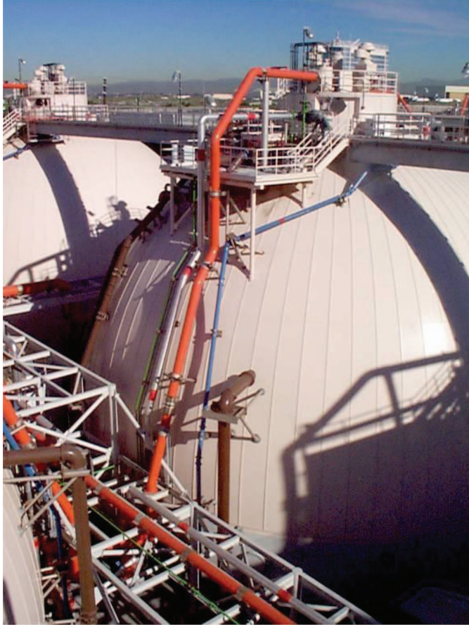
Fig. 12-9. Gas Domes and Platform
