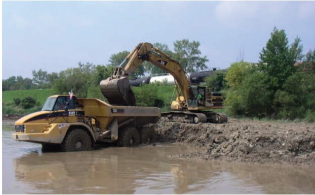
Fig. 5-13. Earthwork (Vulnerable to Flooding)
