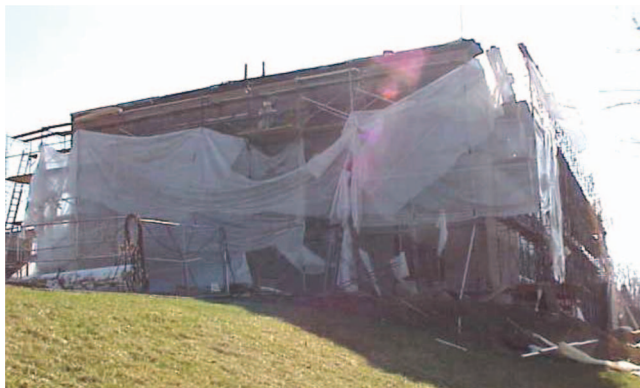
Fig. 5-2. Temporary Building Enclosure Damaged by Wind
