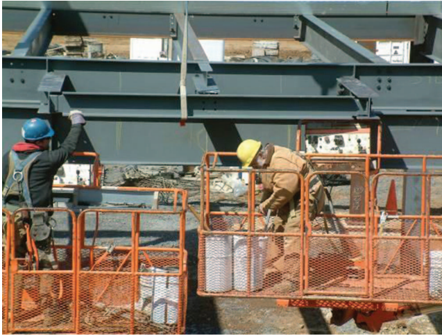
Fig. 11-4. Subcontractor Engaging in an Unsafe Rigging Practice
