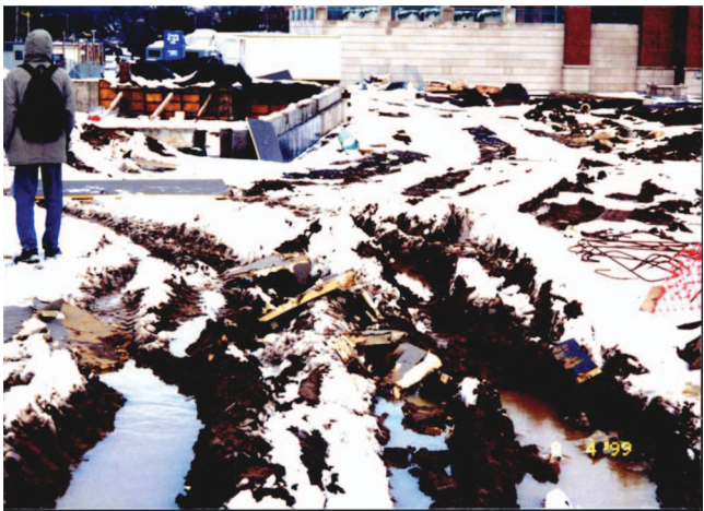
Fig. 5-4. Muddy Site Conditions Caused by Snow and Failure to Seal Exposed Areas
