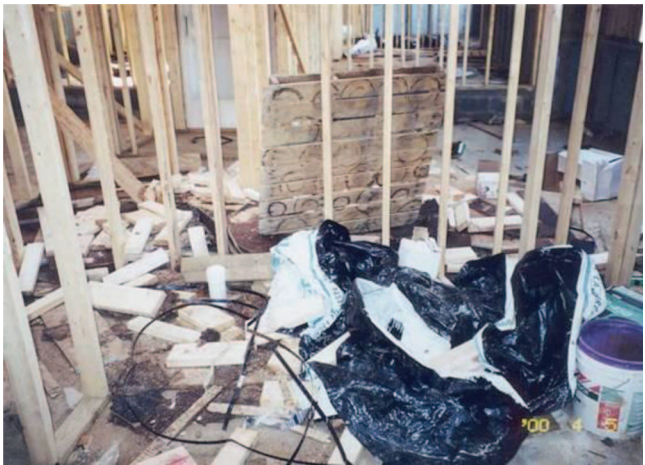
Fig. 6-20. Poor Housekeeping in a Work Face Area
