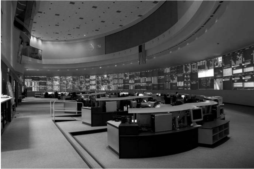
Fig. 14.5 AT&T Global Network Operations Center
